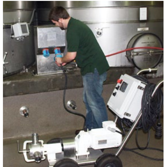
Ryan Carson, Cellar Man at ZD Wines uses Meltric DECONTACTOR plugs and receptacles for their immeasurable amount of safety and plug-n-play capability, which reduces time spent connecting and disconnecting portable pump carts.
